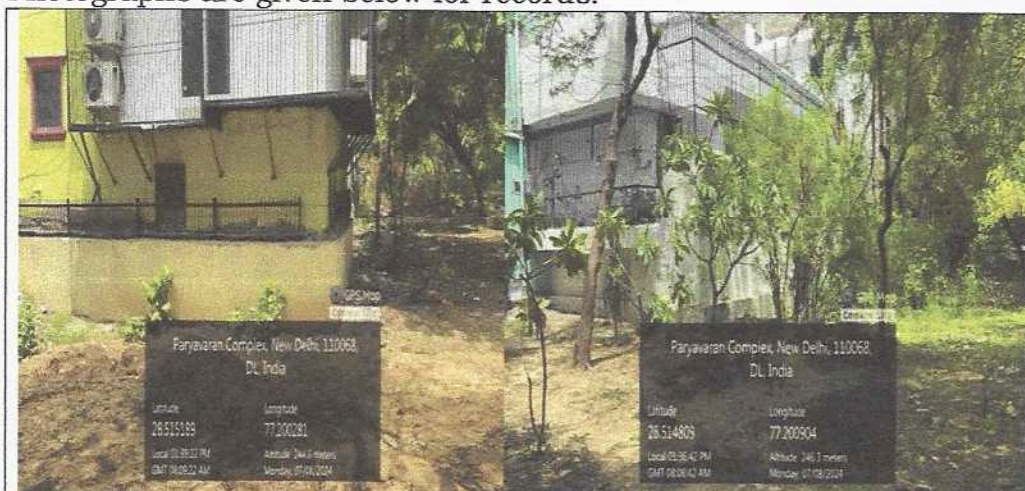
Encroachment of the boundary of Park with overhanging balconies and as support for encroachment structure
