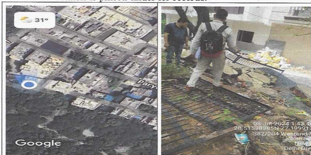
Damaged Boundary wall of the park
